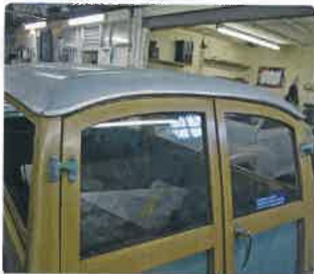
9 The roof panel really shouldn't have been painted before being fixed in place and as you can see, the edges are now in primer after the roof was adjusted to fit properly last month.
