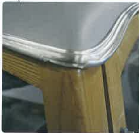
10 The drip rail and moulding covering the nail heads should be in body colour, so will be painted when the roof is repainted.
